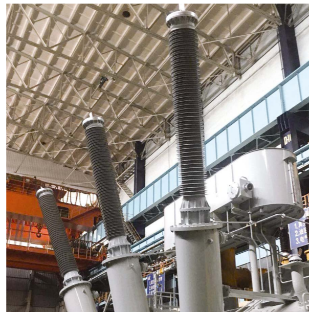
550kV 变压器套管安装在变压器上进行出厂试验 Installation of 550kV transformer bushing on the transformer for Routine test
